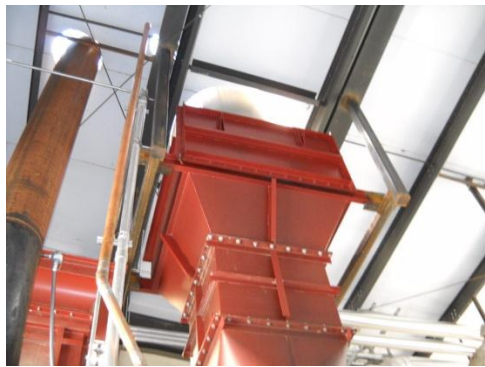
SCR on 50,000 PPH Firetube Boiler
