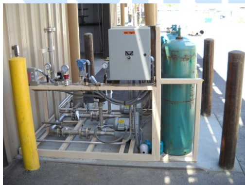
Ammonia Delivery Skid
